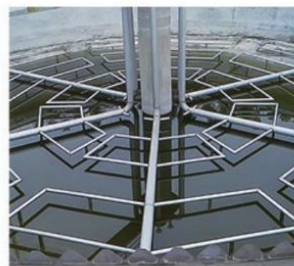
穿孔曝气机 Perforated aerator
